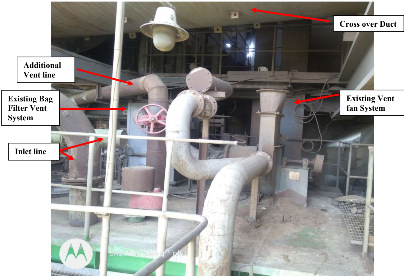
Bed Material Silo-top view
