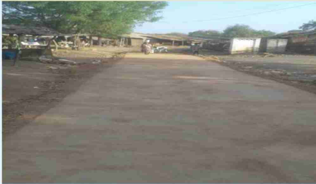
Construction of RCC Road at Village Nani Naroli, Taluka Mangrol, District Surat
