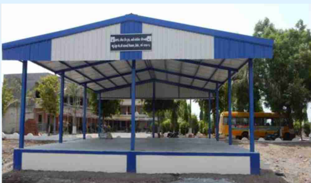
Construction of Multi purpose shed at village Ushker, Taluka Mandvi, District Surat
