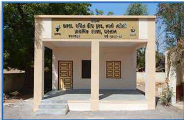
Construction of Class Rooms, Primary School at Village Vastan, Taluka Mangrol, District Surat
