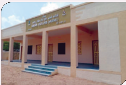
Construction of Classrooms (3 Nos.) for Primary School at Village Shah, Taluka Mangrol, District Surat
