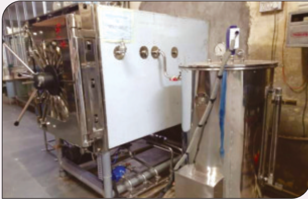
Autoclave machine for sterilization New Civil Hospital, Surat
