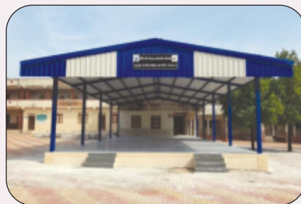
Construction of Multipurpose Shed for High School at Village Nani Naroli, Taluka Mangrol, District Surat
